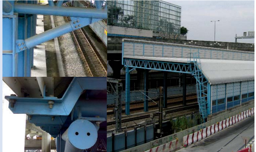
MTRC Airport Railway West Kowloon Section Noise Enclosure 機鐵西九龍隔音屏
