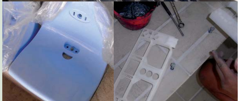
Improvement to Kowloon Park Swimming Pool 九龍公園室內游泳池改善工程
